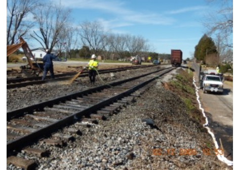
At-Grade Crossing Diesel Release
