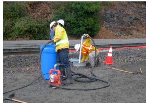
Fuel Flushed and Degraded from Trackbed with HC-2000
