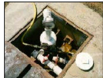
HC-2000/BioSparge Injection Well at Gasoline GUST Trust Fund Reimbursed Site
